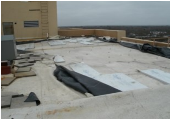
Ocean Cove's roof endured up to 70 MPH winds from Super Storm Sandy
