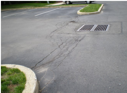
Poor surface pavement conditions
