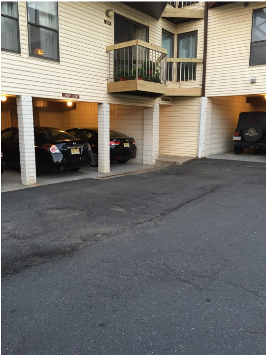
Area of ponding which resulted in disturbed asphalt pavement.
