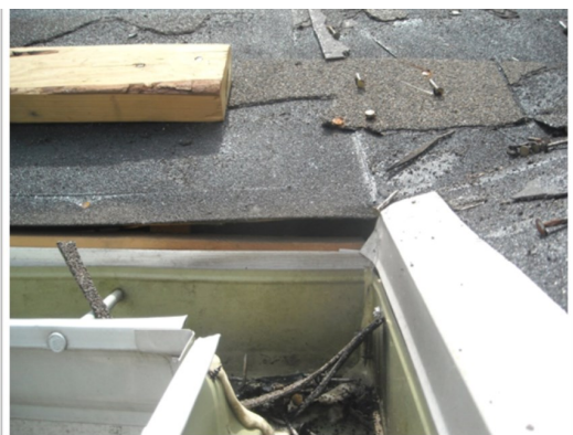
Example of structural damage of the stone facade and gaps between fascia boards at roof sheathing as a result of improper installation
